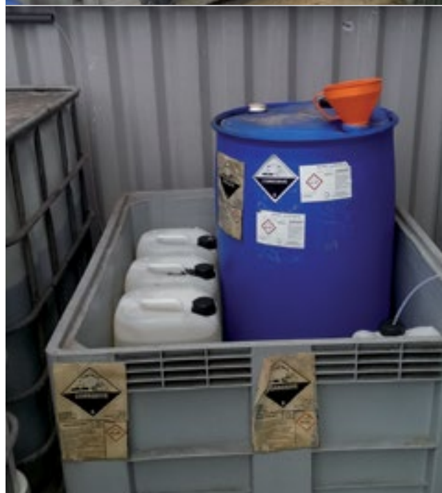
Figure 9. A typical automated acid injection system on a nursery (top) and associated acid storage (bottom)
