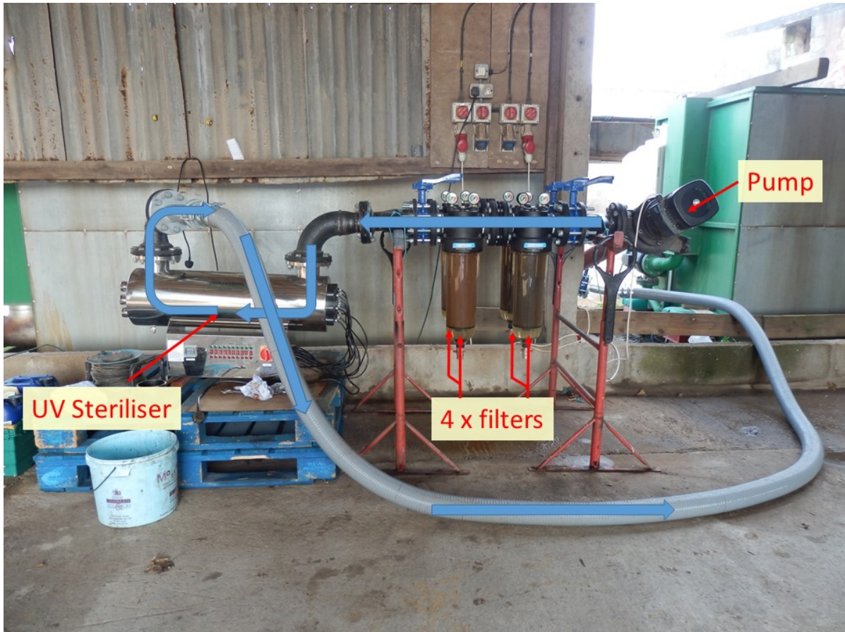
Figure 1. Retro-fitted filtration and UV system at Carwin Farm, Cornwall
